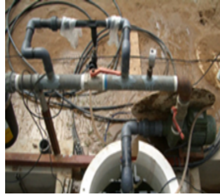
Fig. 4: Pump of the cold tank
